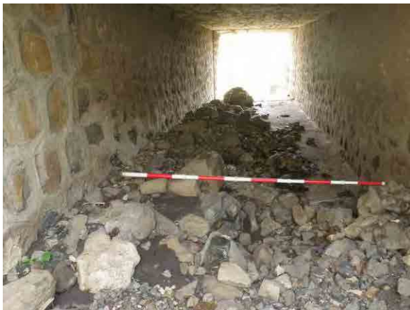
Photo 3. 9.7 Sediment which is deposited in the box culvert installed under the road (1.6m high and 2.0m wide)
