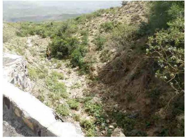
Photo 3. 9.22 Entire picture of MS008 (downstream from the road; gullies develop)
