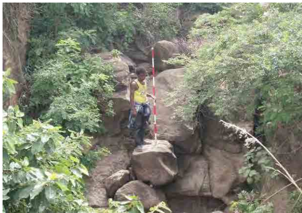
Photo 3. 9.65 Large rocks near the box culvert
