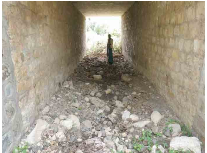
Photo 3. 9.30 Box culvert installed under the road (sediment deposits cover the entire inside)
