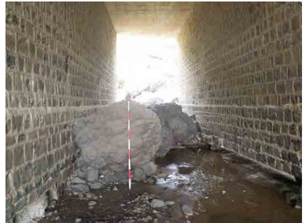
Photo 3. 9.109 Large rock in the box culvert
