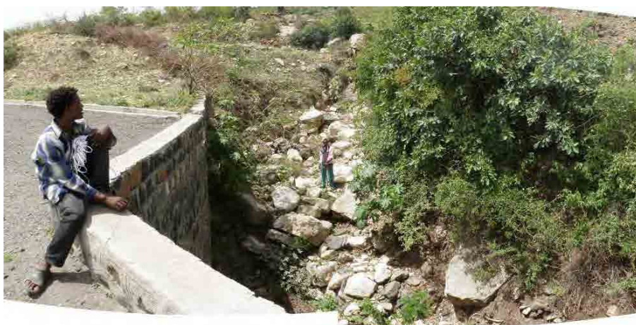
Photo 3. 9.31 Entire picture of MS011 (upstream from the road; no water flow confirmed)
