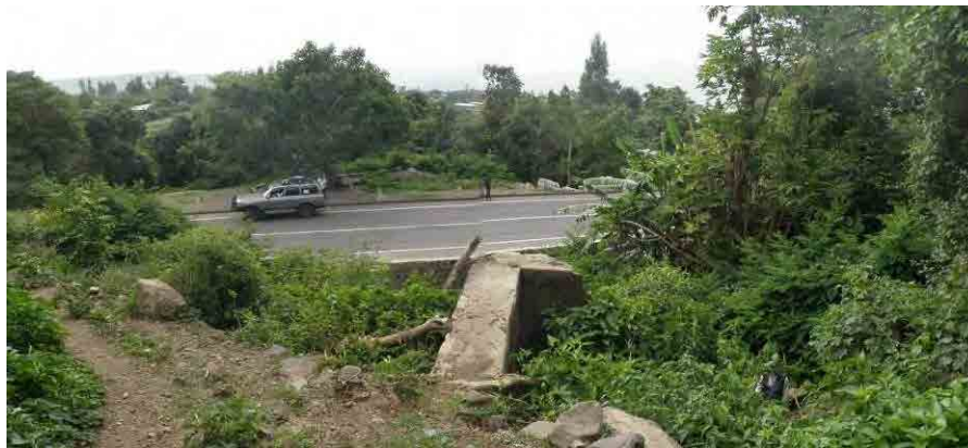
Photo 3. 9.88 Damaged dam (taken from the upstream of the road)
