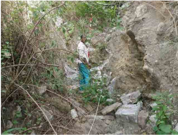
Photo 3. 9.56 Channel upstream (channel bank erosion)
