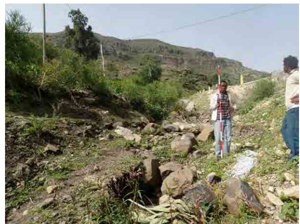
Photo 3. 9.8 Channel upstream (located at the drainage of traversing drainage systems and road)
