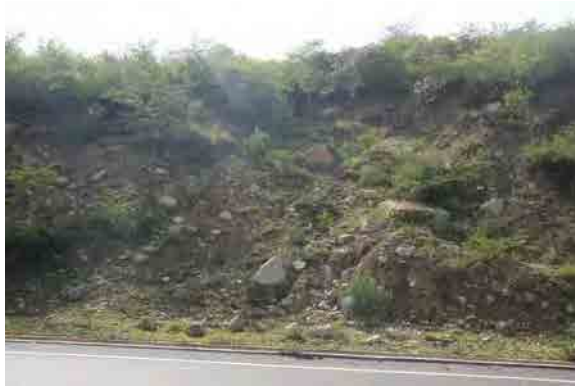
Photo 3. 8.15 Detached rocks distributed on the slopes
