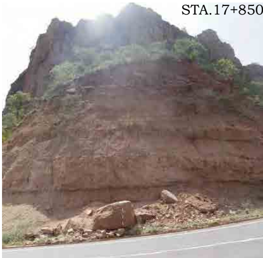
Photo 3. 8.21 Fallen rocks distributed along the roadside
