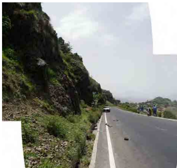
Photo 3. 8.37 Fallen rocks from the cut slope
