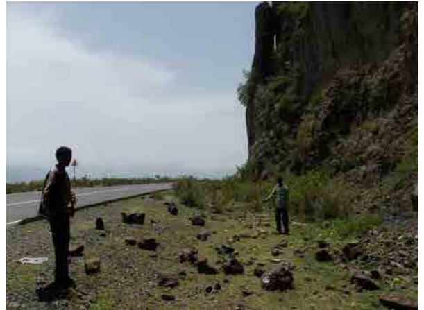
Photo 3. 8.12 Fallen rocks distributed on the slope bottom
