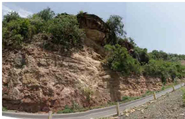
Photo 3. 8.29 Overhanging cut slope (around STA.21+300)
