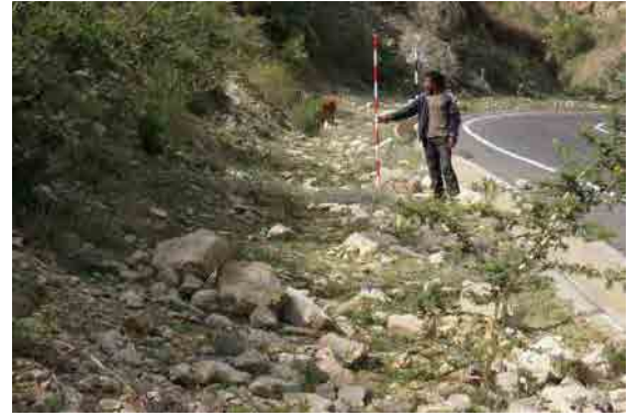
Photo 3. 8.16 Fallen rocks deposited at the slope bottom
