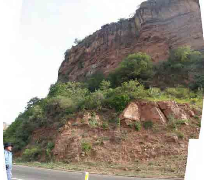
Photo 3. 8.24 Cut slopes softened due to weathering
