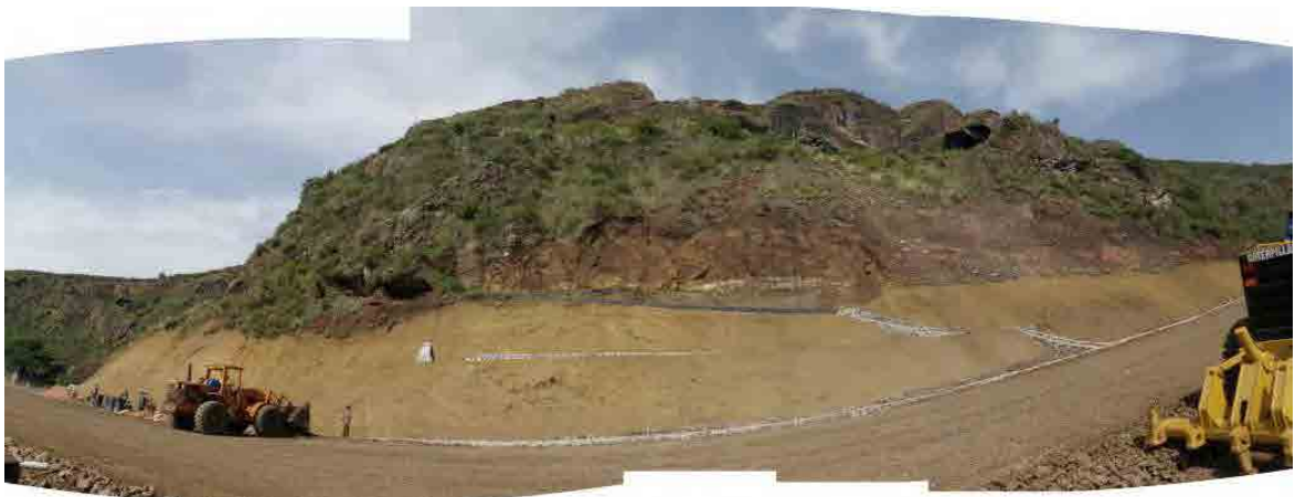
Photo 3. 8.3 Construction work being done by ERA (wastewater work construction and roadbed construction, STA.0+88 – 1+880)
