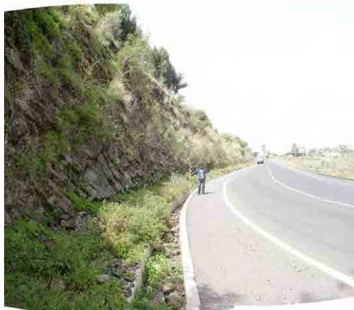
Photo 3. 8.39 Fallen rocks from the cut slope (the section end side was taken from around area STA.35+350)
