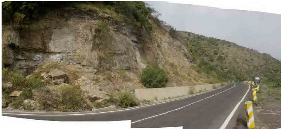
Photo 3. 8.19 Retaining wall on the section end side (fallen rocks are distributed on the retaining wall side)
