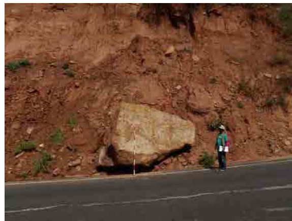
Photo 3. 8.27 A fallen rock 2.5m in diameter
