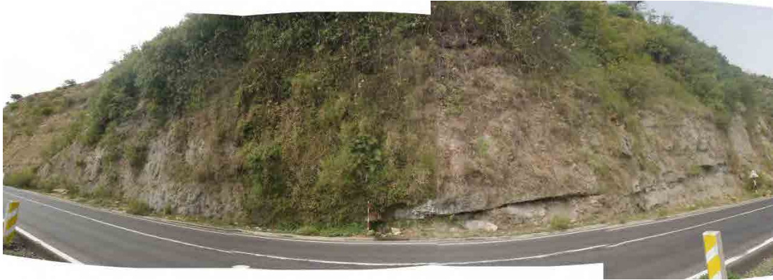
Photo 3. 8.18 Natural slope between both of the retaining walls (a spring can be observed at the layer border)
