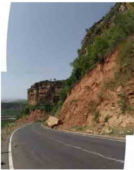
Photo 3. 8.26 Fallen rocks around STA.20+800m
