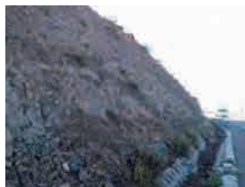
Photo 5.4.10 Rockfall from a Cut Slope
