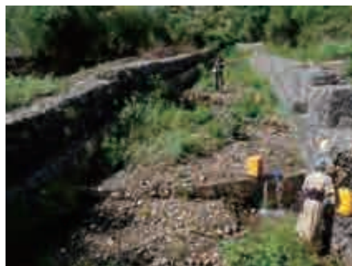
Photo 5.4.6 Gabions along the stream banks
