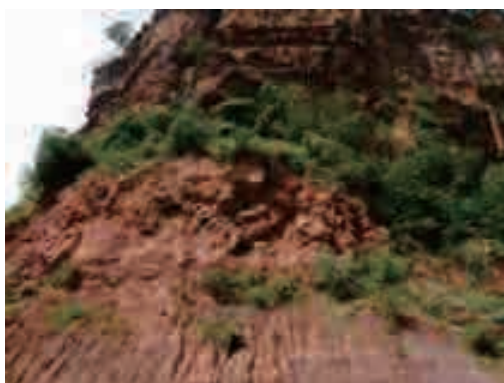
Photo 5.4.7 Fall-off Type Rockfall
