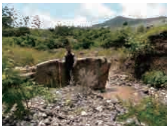
Photo 5.4.13 Damaged dam sleeves
