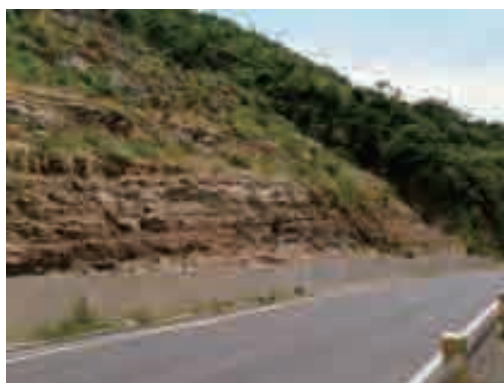
Photo 5.4.1 Rockfall Protection Wall
