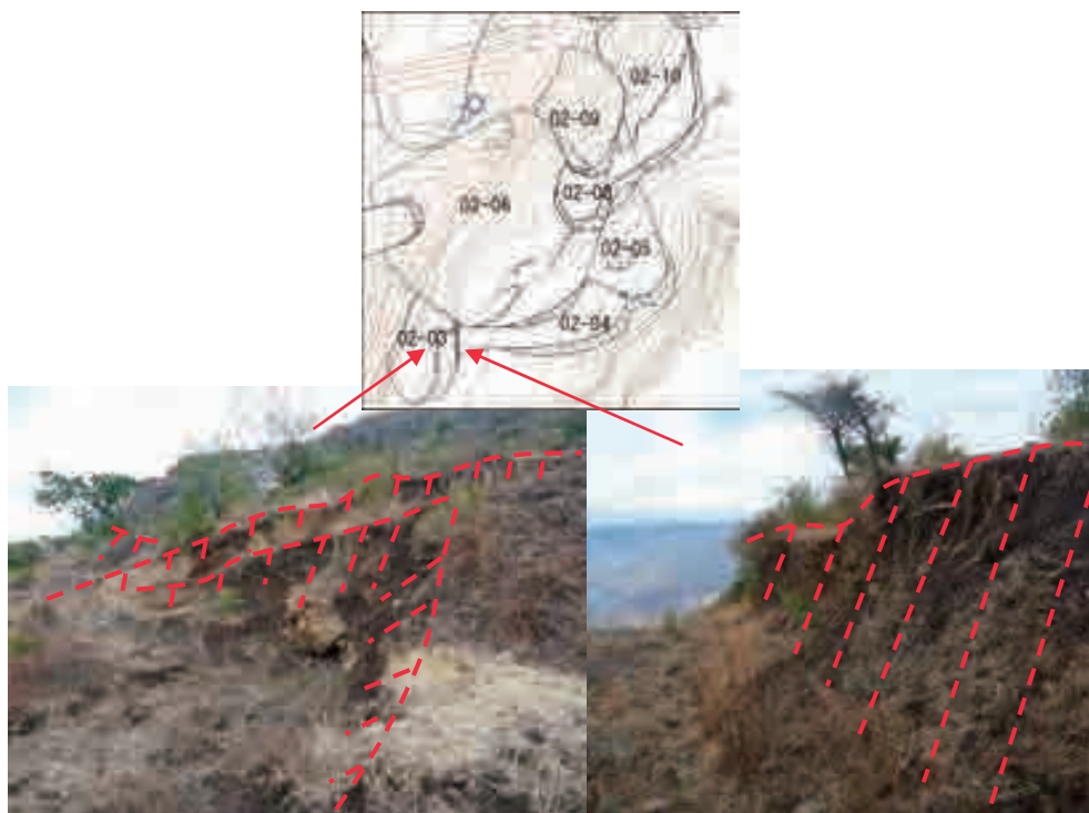
Figure 4.3.18 New Cracks at the Head of L/S02-03
