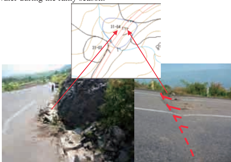
Figure 4.3.31 Deformation of the road at L/S31-04
