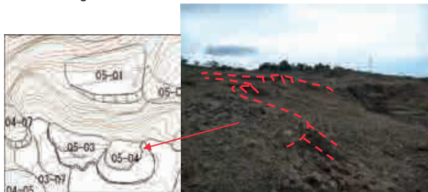
Figure 4.3.22 New Cracks at L/S05-04
