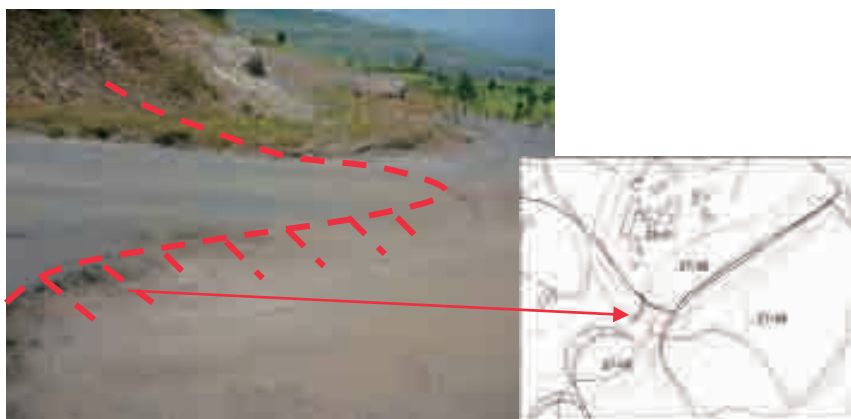
Figure 4.3.27 Deformation by the extension of L/S27-04
