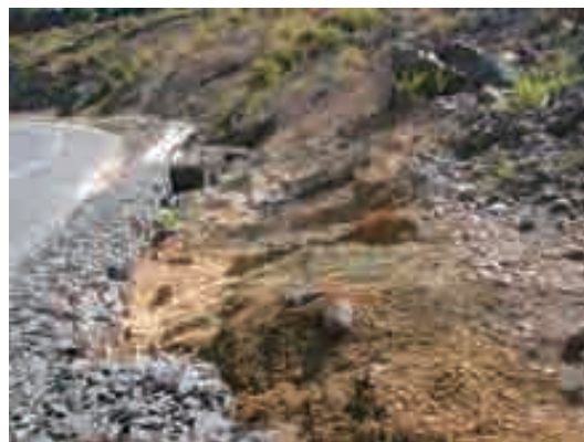
Photo 4.4.16 The layer is very soft and erosive, which trigger slope collapses
