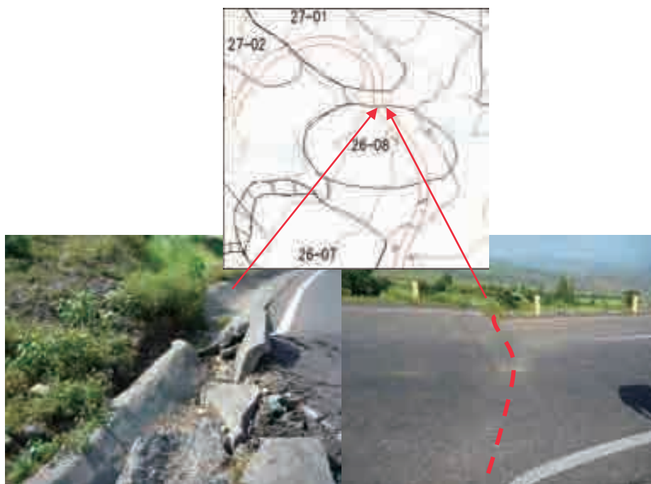
Figure 4.3.26 Side crack of L/S26-08
