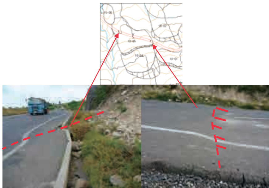
Figure 4.3.24 Deformation of the road by L/S10-05
