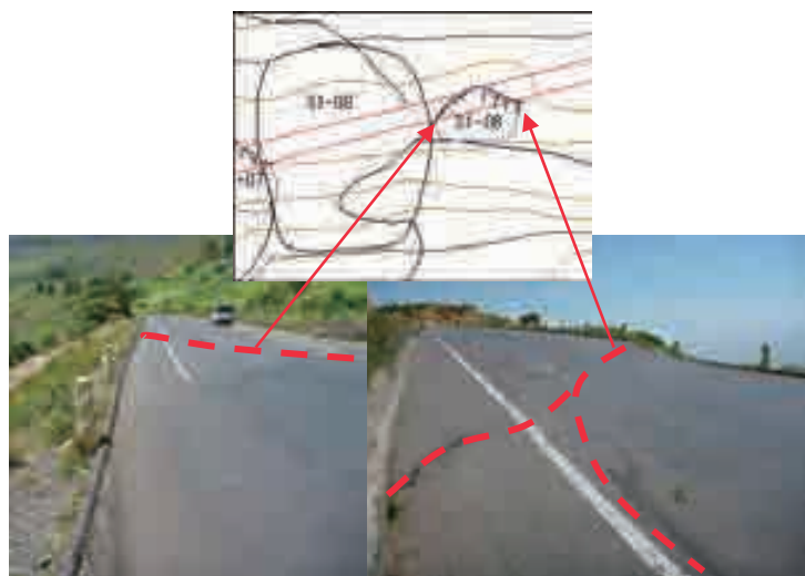
Figure 4.3.33 Deformation of the road at L/S31-08
