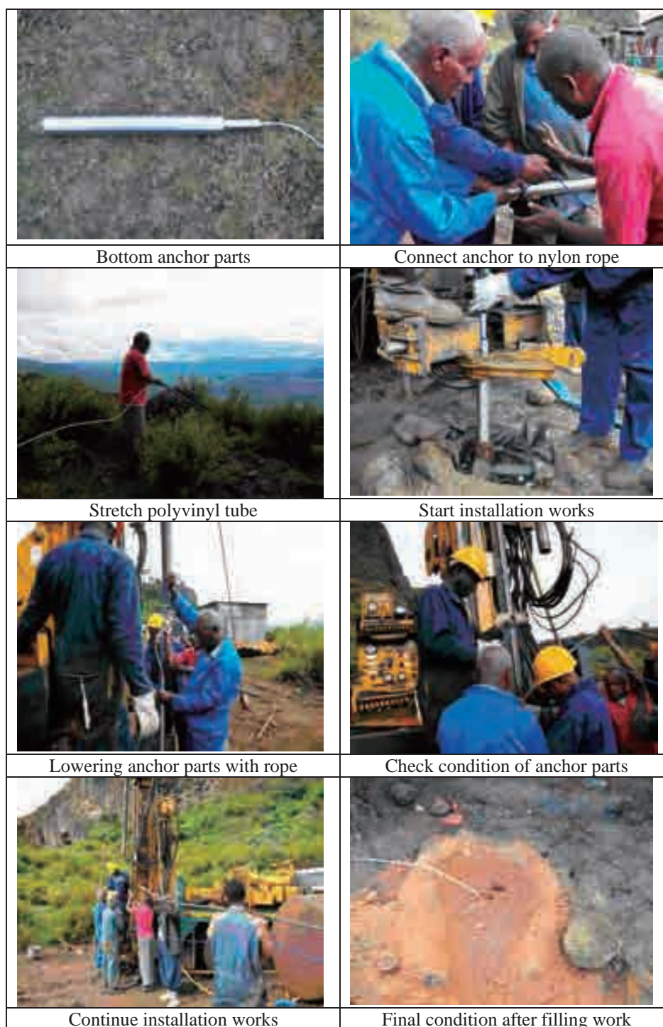
Photo 3.7.2 Field photograph for the borehole extensometer
