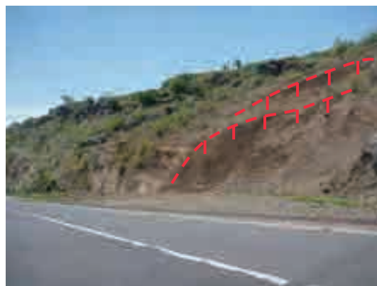
Photo (4) Small collapses on the mountain side of the toe of the L/S05-1 (1) Multiple small collapses are occurring on the slope.
