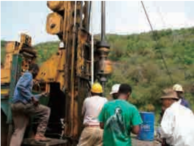
Technical transfer on drilling. Installation of casing pipes for inclinometer, 12 th Jul. 2011
