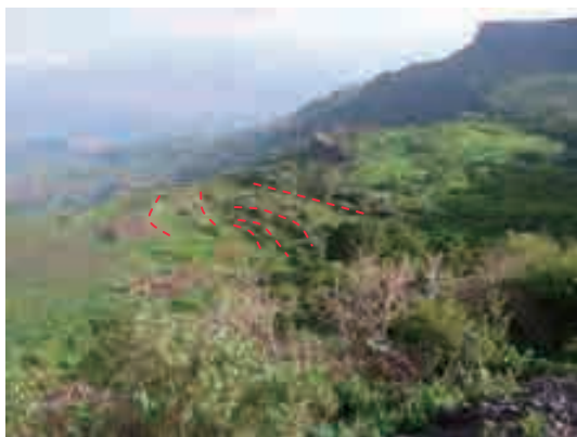
Photo (1) Distant view near the boundary of the lower part of L/S00-1 and L/S00-5 Wrinkle-like irregular land features running in parallel. Deformation seems to be occurring in L/S00-5 due to movement of L/S00-1.
