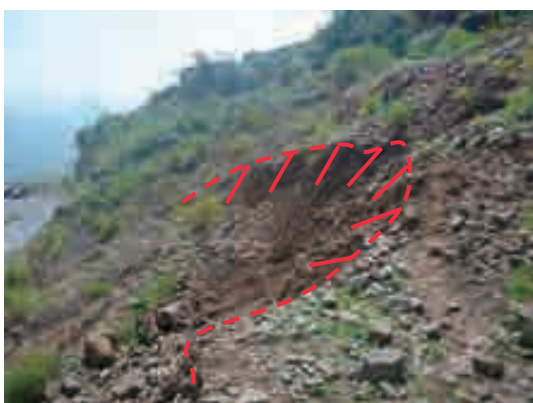
Photo (5) Small collapses on the mountain side of the toe of the L/S05-1 (2) Small collapses as viewed from inside the block.
