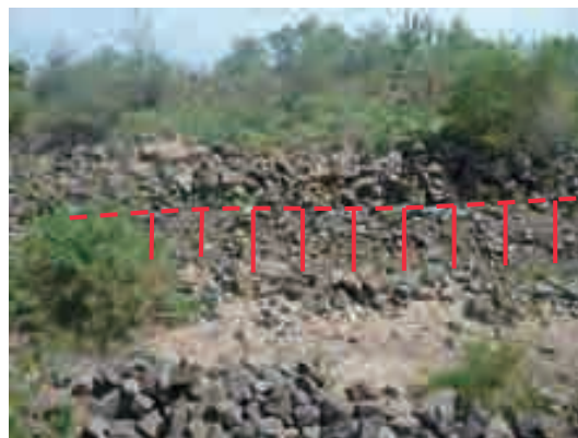
Photo (2) Expansion of the cracks along the channel in the L/S05-1. The blue vinyl sheet that was covering the old channel has been torn, so it can be considered that cracks are expanding along the old channel.
