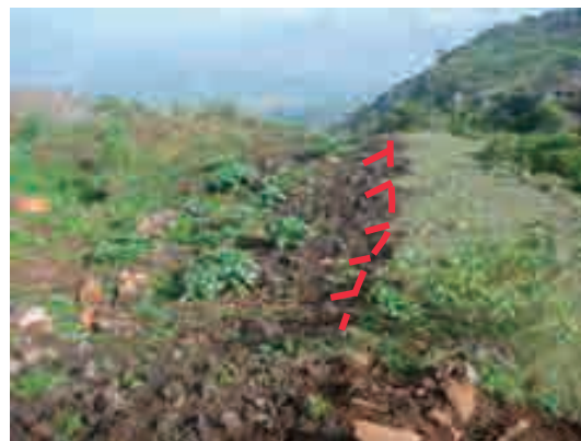
Photo (2) Lateral cracks on the L/S00-2 block Multiple small cracks are opening on the right flank of L/S00-2.
