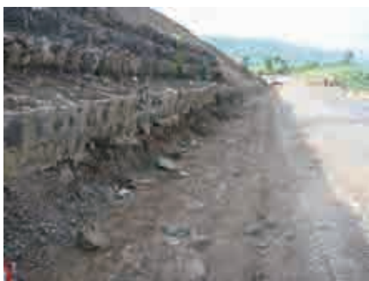
Photo (9) Top of the L/S27-2. The road surface is sinking at the top of the block, causing a maximum difference in altitude of 1m from the former roadside channel. It can be seen that the top of the block has sunken due to the landslide.
