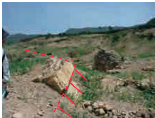
Photo (2) Main scarp and subsidence in the L/S28-3 (2). Cracks whose mountain side is sinking can be seen on the head of the slope. New cracks are continuing from this crack.
