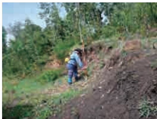
Photo (4) Main scarp in the L/S28-1
