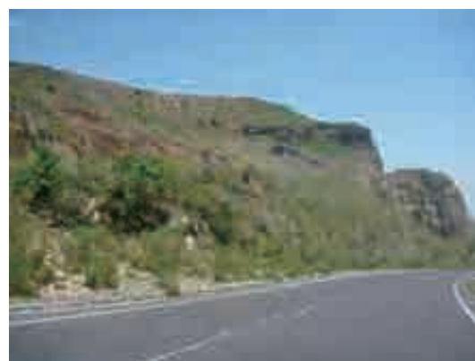
Photo (6) Top of the L/S05-2 The debris area from the L/S05-01 block is considered to be the L/S05-02 block. Cracks indicating a small collapse are occurring at the top of the block.
