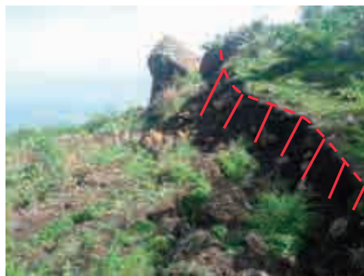
Photo (6) Crack and a fallen rock at the toe of the L/S00-1. A 1 to 2m deep crack with a difference in level is continuing at the lower part of the L/S00-1. Near the center, a large rock had fallen, with the previously buried portion appearing. The strike of the rocks seems to be similar with the one of the L/S00-1.
