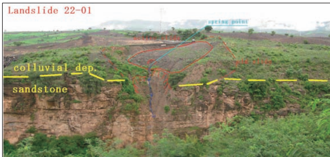
Photo 3.10.1 Landslide 22-01 from opposite side terrace cliff.
