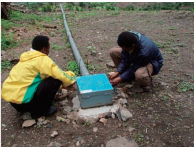
Installed extensometer at the landslide
