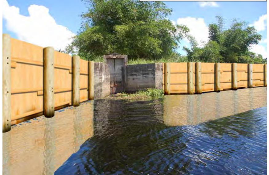
INTAKE facility composition
