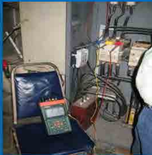
La Sultana Plant
