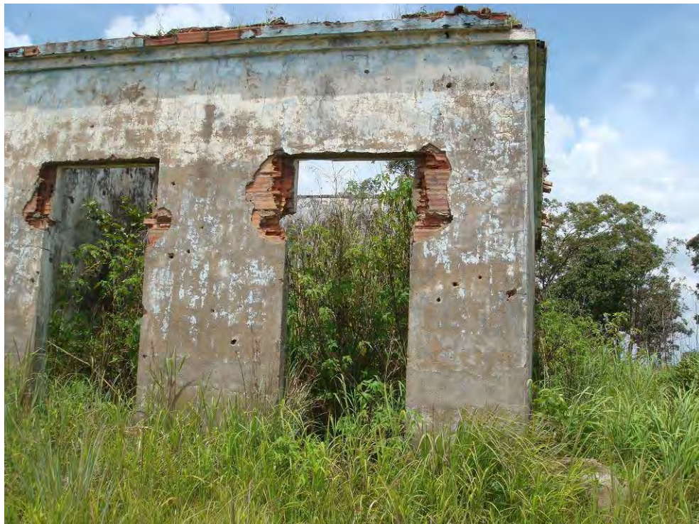
Photo 4.2-2(3) Ruined Bullet Trace in Chimonga Village
