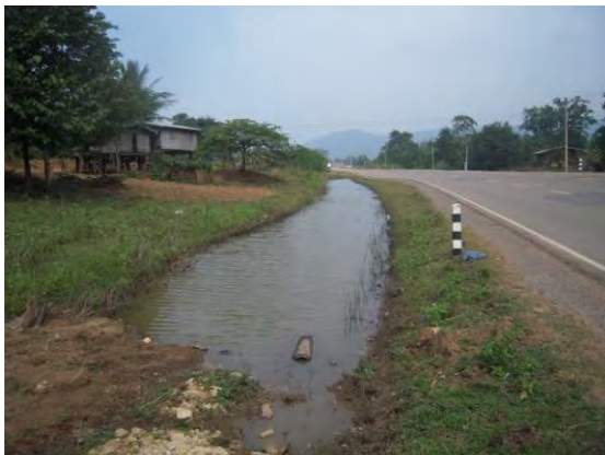
Poor drainage at Muang Phin
