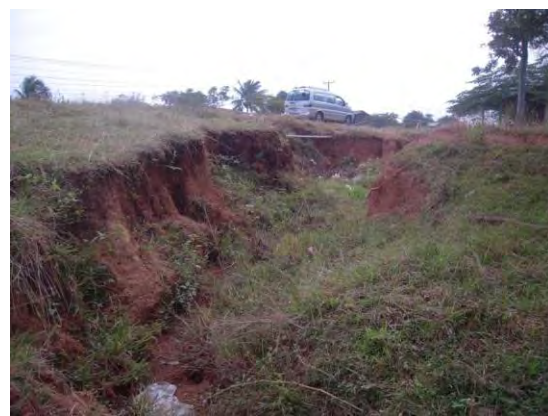
Erosion of ditch
