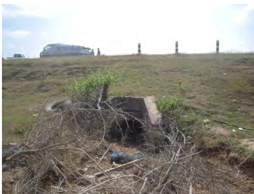
The culvert, which is installed at the lowest point of the area.
