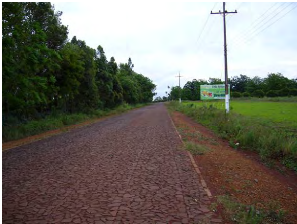
Typical cross-section of the National Road Route 6 - Coastal Road Connection Road (Stone Pavement Section)
