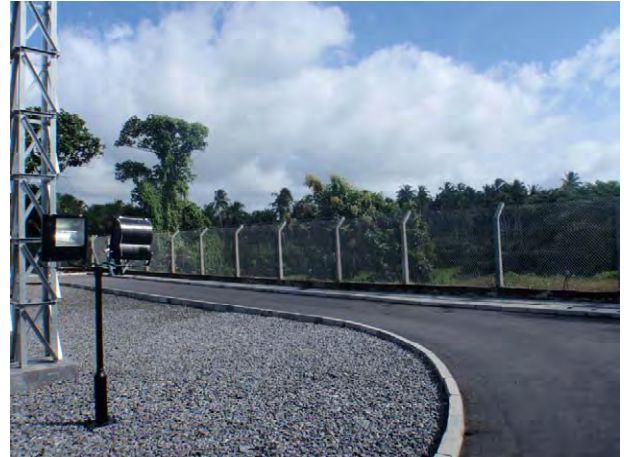
220kV Bus Extension Space in Veyangoda GS
