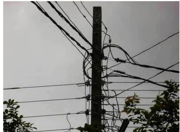
Connection of Low Voltage Lines and Low Voltage Concrete Pole
