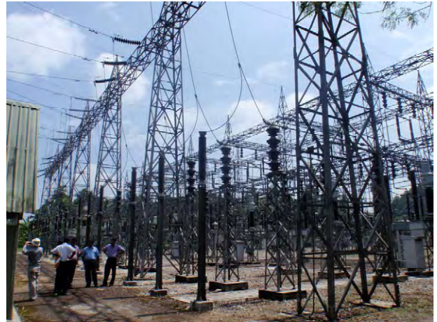
132/33kV Ukuwela Switchyard
