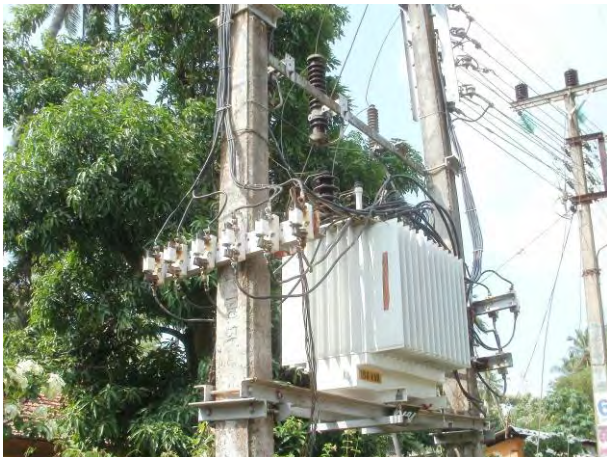
33 kV/400-230 V Step-down Transformer and Low Voltage Lines
