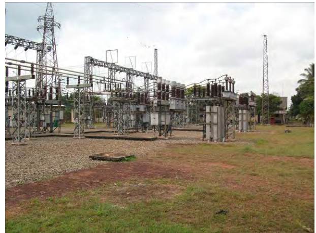
33 kV Switchyard at Biyagama GS
