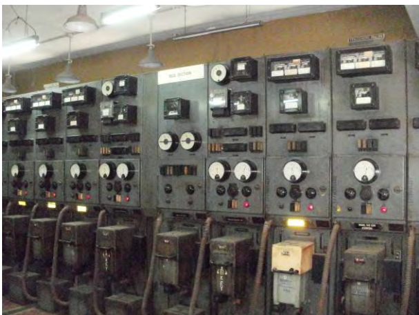
11 kV Switchgear at Colombo-C GS
