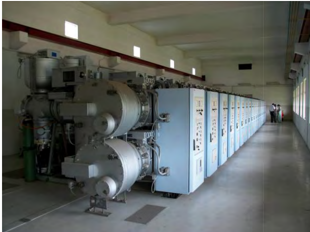
132 kV GIS at Kolonnawa – New GS
