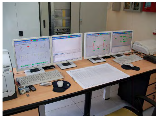
Remote Control System at Bolawatta GS
