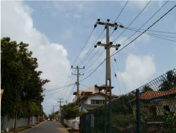
33 kV Distribution Lines
