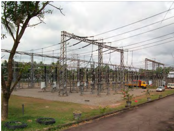
220/132 kV Switchyard at Biyagama GS
