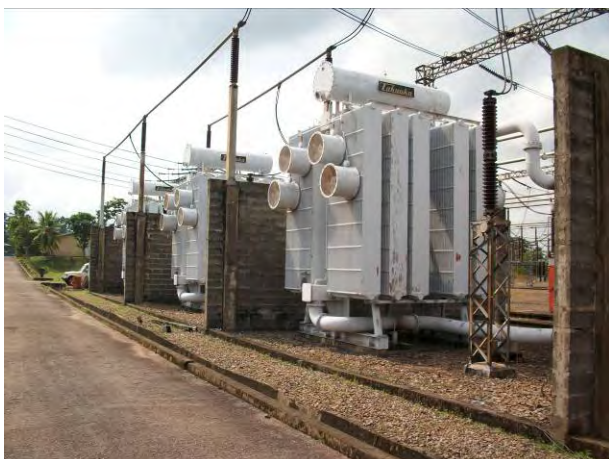
220/132/33 kV Auto-transformer at Biyagama GS
