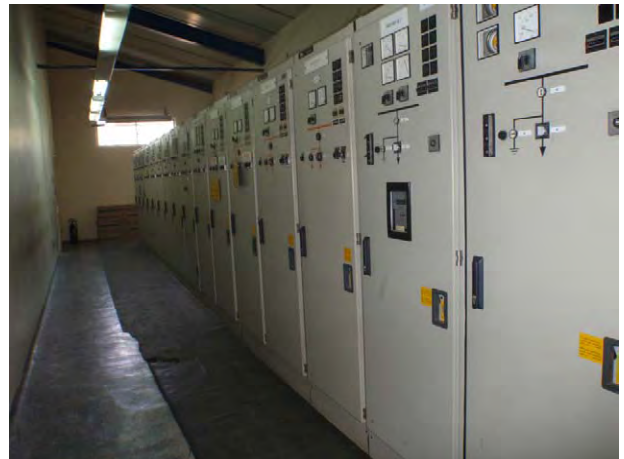
33 kV Switchgear in Kiribathkumbura GS
