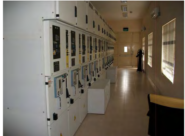
33 kV Switchgear at Pannala GS
