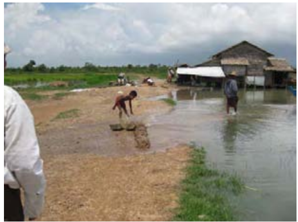
Before Rehabilitation – Polder Dike Overtopping river water into polder during high tide near Hpobe Sluice (August 2010).
