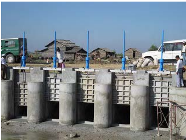
Sluice Rehabilitation Work Under final setting of slide gates at Mayan South Sluice.
