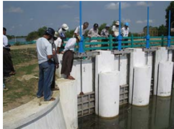
Sluice Rehabilitation Work Completion inspection together with ID, contractor and JICA Team (31 March 2011).
