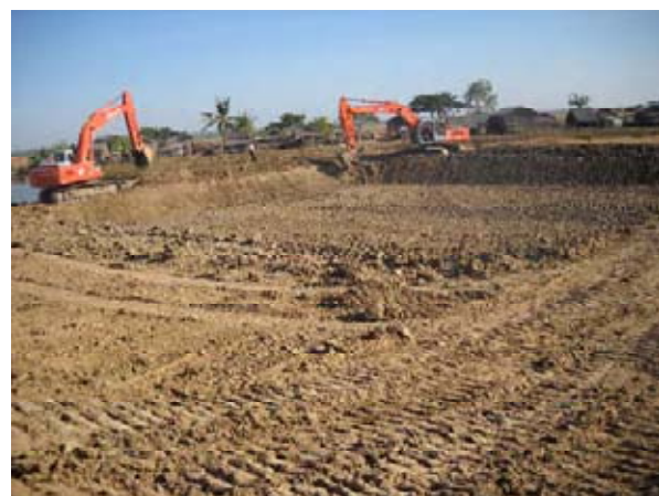
Polder Dike Rehabilitation Work Soil borrow area is set for water pond for villagers use.
