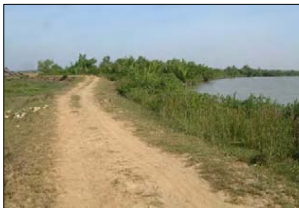
Present Condition of Existing Dike: Small & Low (January 2010, at the time of high tide)
