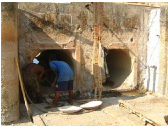
Sluice Rehabilitation Work Just after removal of existing slide gates at Hpobe Sluice.
