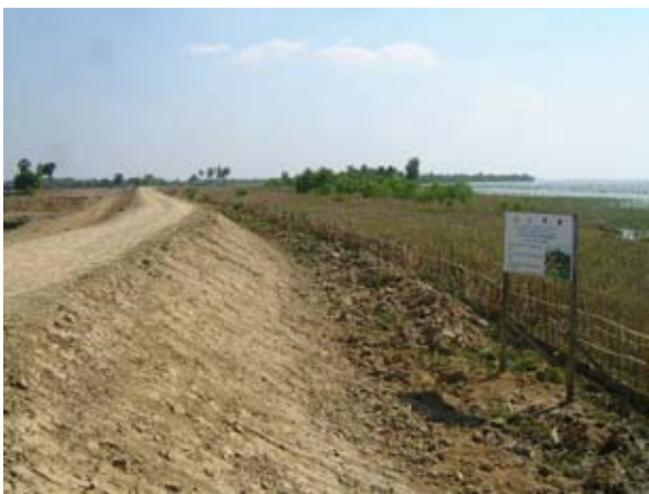
Mangrove Windbreak Project Completed dike embankment and mangrove pilot project site (February 2011).
