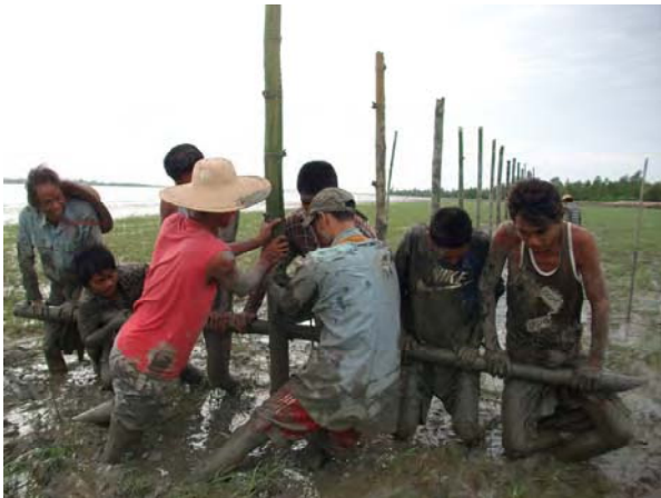
Mangrove Windbreak Project Fence making to protect from tidal wave & river flow (May 2010)
