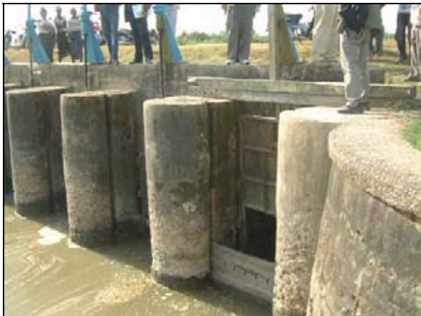
Before Rehabilitation – Sluice Gate Broken slide gate at Danedan Sluice (January 2010).
