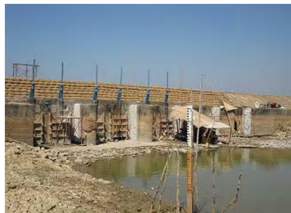
Sluice Rehabilitation Work Under chipping of existing concrete for repair of slide gates at Hpobe Sluice.
