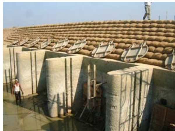
Sluice Rehabilitation Work Just after removal of existing flap gates at Hpobe Sluice.
