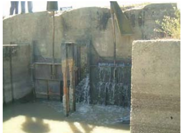
Before Rehabilitation – Sluice Gate Water leakage due to flap gate non-functioned (January 2010).
