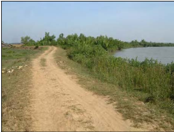
Before Rehabilitation – Polder Dike Common view of polder dike with farmland, mangrove and river (January 2010).
