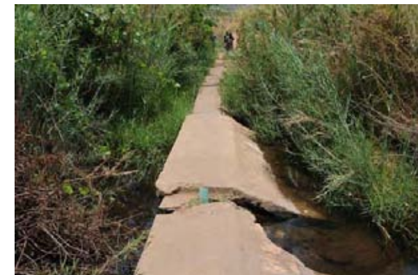
Blocks of the weir body slid down at contraction joints due to settlement of the foundation.
