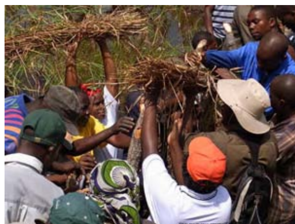
A lot of things are going on at once. Weir construction is definitely a collaborative activity
