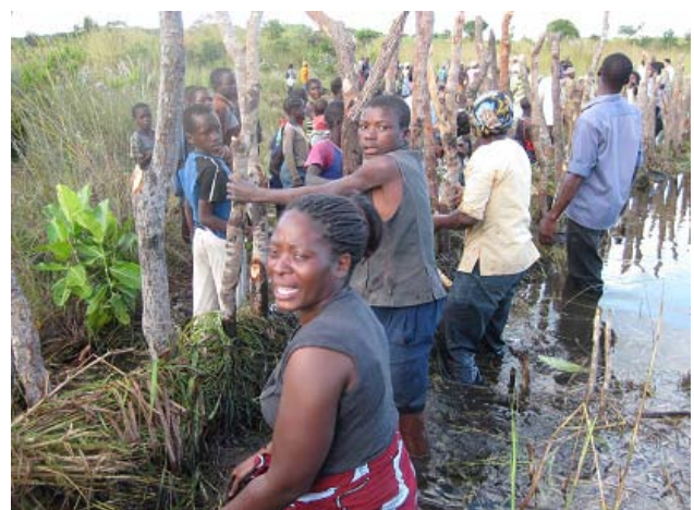
Trainees are constructing the temporary brush dam, made out of locally available materials.
