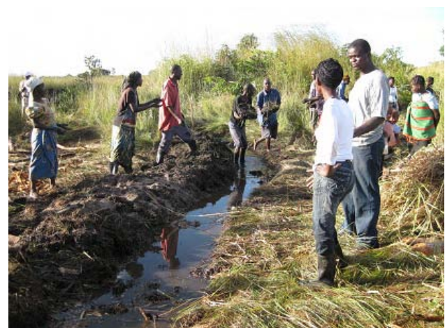
Canal was dug according to the counter set by line-leveling, and the water starts flowing by gravity.
