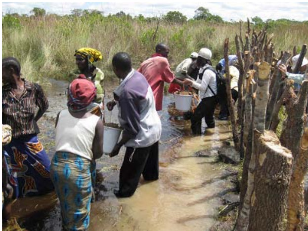
Participants are practicing construction of a temporary diversion weir, putting clay soils beneath the weir body.
