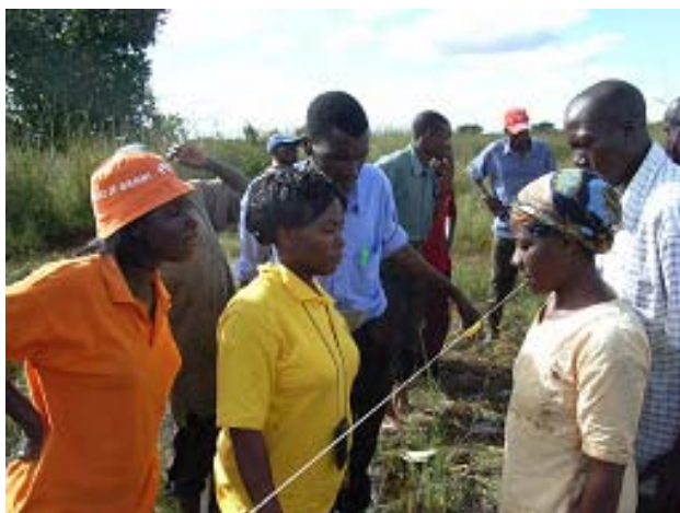
Trainees are reading spirit level hung on the line, getting suitable gradient for canal which can deliver water by gravity.
