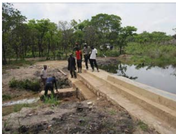
The masonry main body has completed. The persons concerned such as the community members, TSB staff, and skilled labors are finally checking the details of facility. (As of early in November, 2010)
