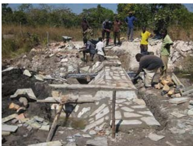
The masonry type of weir has been almost piled up on the Kasakalabwe stream, Mporokoso district (as of mid July)
