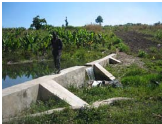
Of late years, many permanent concrete diversion weirs were constructed as a part of government program. (June 2009, Mungwi District)
