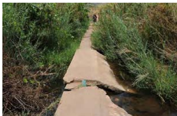
Blocks of the weir body slid down at contraction joints due to settlement of the foundation.
