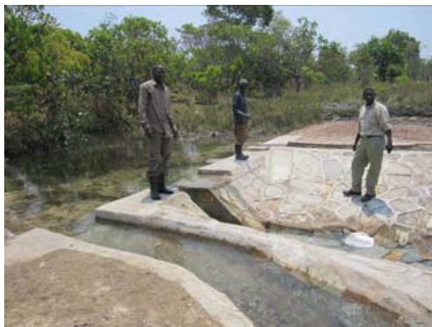
The permanent weir newly constructed has started delivering the irrigation water to the farm land. (As of the end of September 2010)
