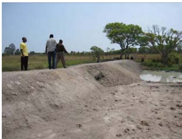
The main body of small-scale earth has been piled up to the level planned. (As of the beginning of November 2010).
