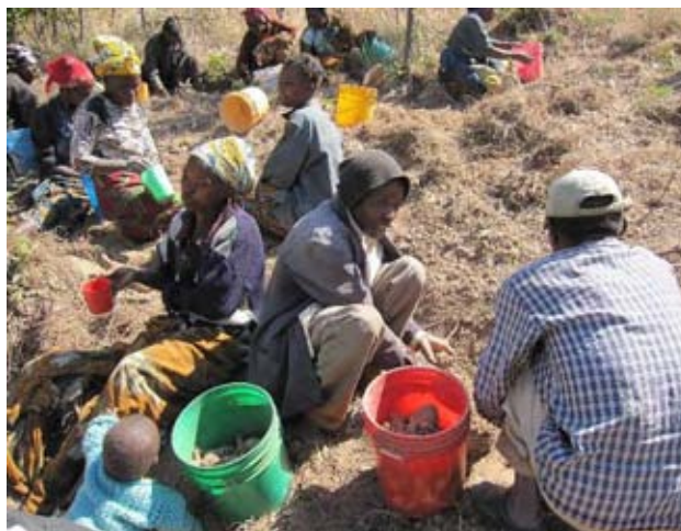
The scheme members are collecting stones for making concrete as preparation work to next stage. (Malashi site, as of the end of June, 2010)
