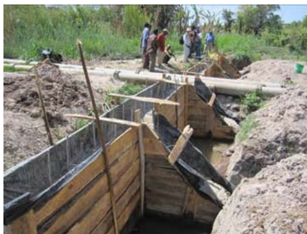
The construction reached the final stage to place concrete to last layer. After that, the construction was successfully finished and then the weir has started supplying enough water to irrigated plots being cultivated by 53 farmers.
