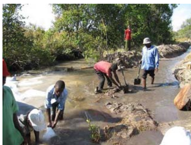
The participants are constructing the de-watering furrow which will be about 100 meter in length. They planned to complete this work within 10 days (Chibolya site, as of beginning of July, 2010).
