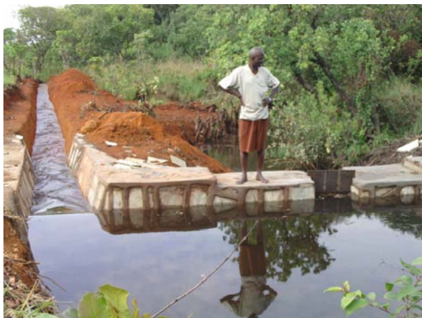
A masonry type of weir constructed under 2010 pilot project has started supplying the irrigated land with water (As of mid-November 2010).
