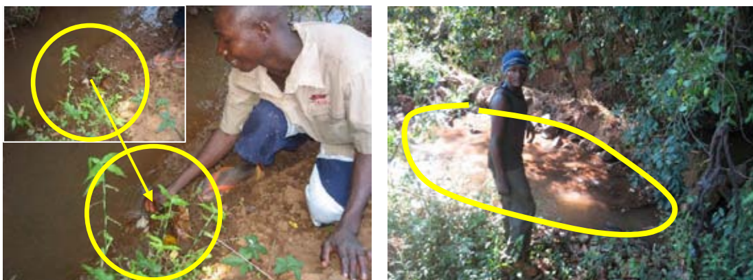
Unlined furrow requires much repair works to avoid water leakage/seepage. In order to plug the holes in the furrow, plenty of soils scrapped of from the ground are used and then downstream of the river is disturbed by the soils flowing out through the holes. (June 2009, Mbala District)
