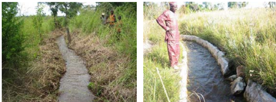
Left: In the case of unlined furrow, the more the length of furrow is longer, the more water leakage becomes much. Right: The farmers try to repair damaged portion in the furrow by using locally available material like soil, stones, and etc. except cement due to financial reason. The maintenance works should be carefully carried out to find signs of damages in advance. (June 2009, Mungwi District)
