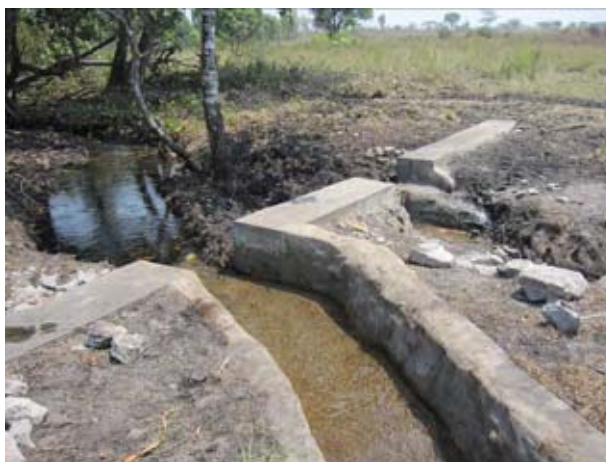
The masonry type weir constructed by Chaiteka community people under the supervision of Luwingu TSB staff. The members now enjoy irrigation farming with the water diverted by the new permanent structure. (As of the end of September in 2010).
