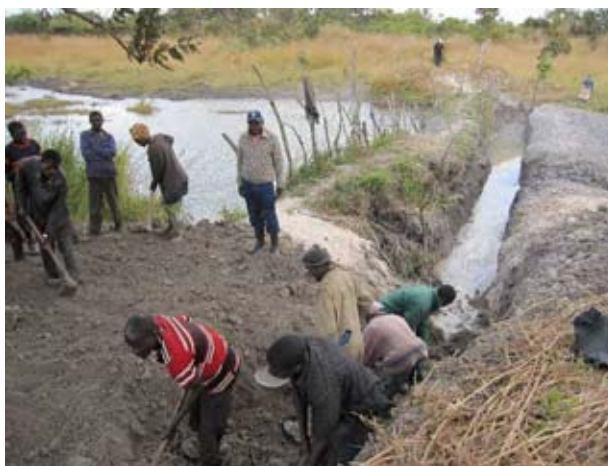
The participants are digging core-trench of the small earth dam. (As of mid-July 2010).
