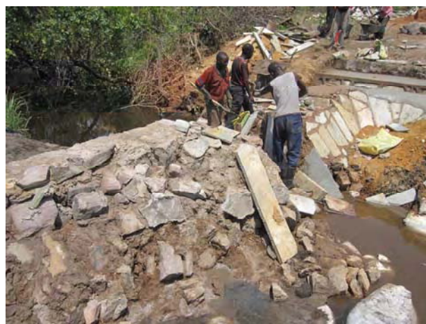
The permanent weir construction was carried out in collaboration with the community people and some skilled labors (As of the end of October 2010).
