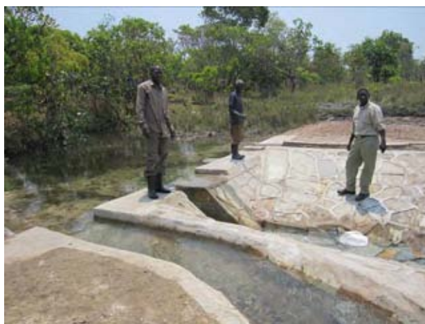
The permanent weir newly constructed has started delivering the irrigation water to the farm land. (As of the end of September 2010)
