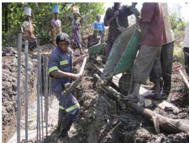
The construction stage is to place concrete for foundation of the weir (Nseluka site, as of mid July).
