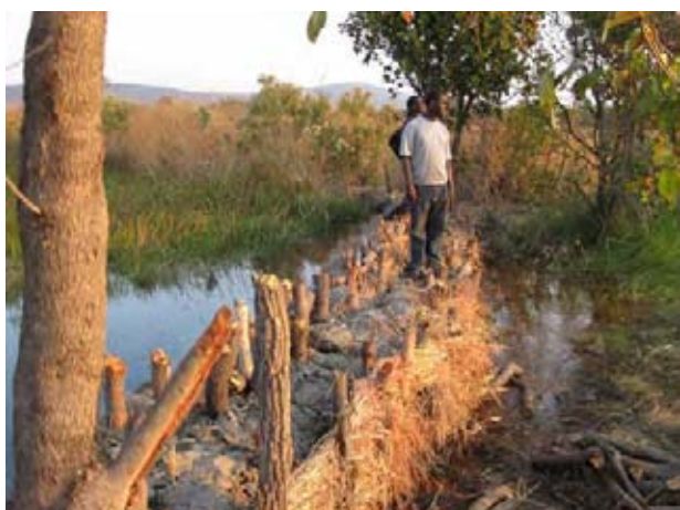
A double-lined simple weir: two lines of single weir are installed in parallel and clay soil is fulfilled in between the two, by which seepage can be minimized and thus water level can be raised easily.
