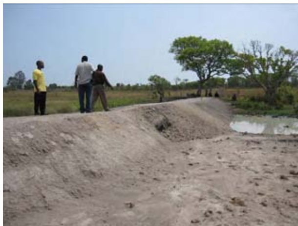
The main body of small-scale earth has been piled up to the level planned. (As of the beginning of November 2010).
