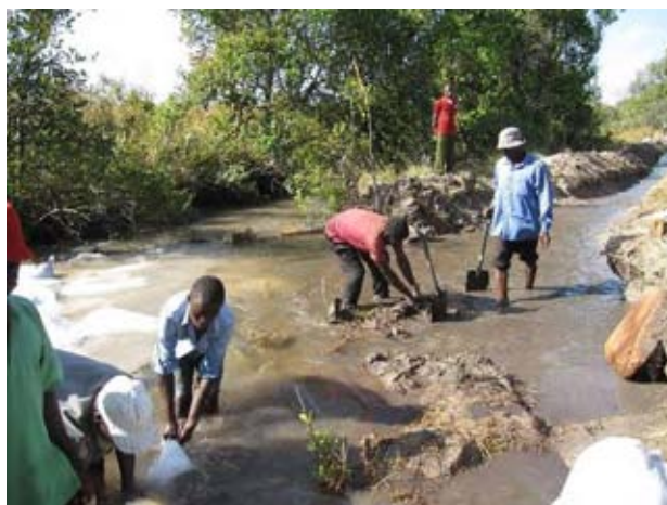
The participants are constructing the de-watering furrow which will be about 100 meter in length. They planned to complete this work within 10 days (Chibolya site, as of beginning of July, 2010).
