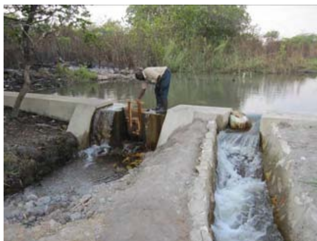
The weir equips a sand sluice gate (Center) from environmental aspect, which is expected to work to flush the sand accumulated in the water pond and to let a small fish go upstream. (As of late in September 2010)
