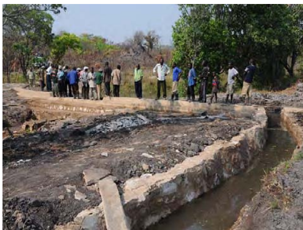
An upgraded permanent weir in Chibolya site, Kawambwa, Luapula Province (length 24m and height 2m): with this weir, more stabilized water is now running in the concrete-lined furrow.
