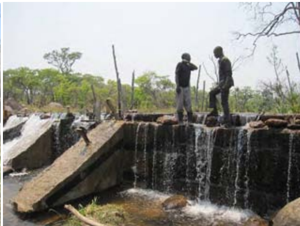
In year 2010, by improving the remaining temporal parts, all the parts of the weir has at last been graded up from temporal to permanent. (As of late in September, 2010 )
