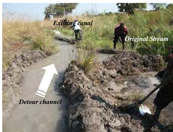
Detour channel is providing water to the existing canal. With this arrangement, dry season irrigated agriculture cannot be interrupted even during the construction of permanent structure.
