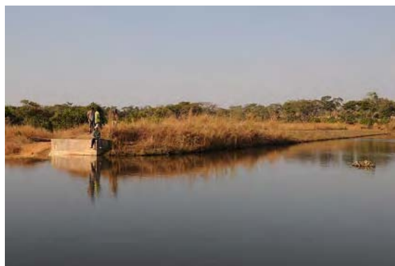
Large man-made earth dam with the length of 206m and the maximum height of 6m. It stays irrigating only 2.5 ha as of 2010.
