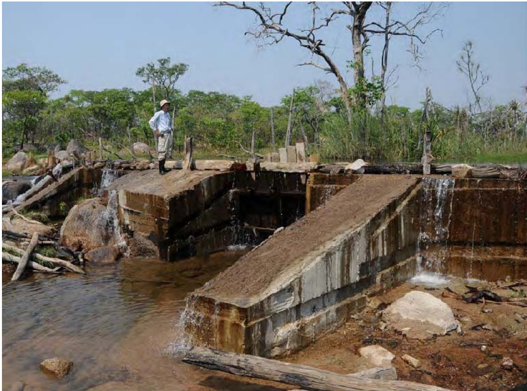
An example of permanent type weir which was upgraded from a simple weir in Mansa district, Luapula province: this 44m-width weir was originally constructed only with timber and clay soils, and was upgraded to this concrete weir. Cement and iron bars were provided both by beneficiary farmers and JICA, and technical assistance had been provided by provincial and district TSB officers.
