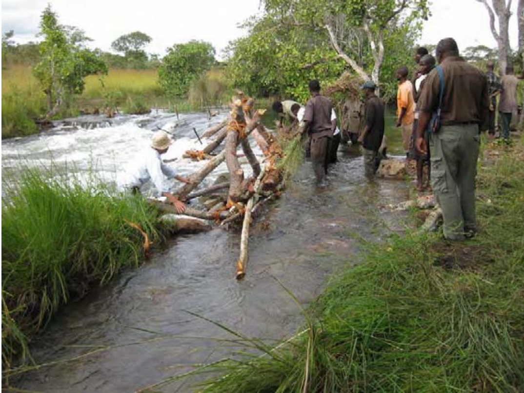
Farmers are constructing a trigonal-prop type weir, the most complicated weir amongst all types of simple weirs promoted in the Study. Assemble pyramidal structures with timbers and put them across the river at about 3m intervals and the weir will be completed after reinforcing with grasses and clay soil. This type of weir can be constructed even on rocky foundation where wooden piles can not be transfixed.
