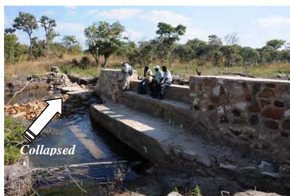
Kapako diversion dam; right side of the weir body collapsed during a flood in late 2008.
