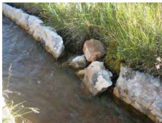
A part of wet-masonry wall is breached; water running away (June 2009, Mungwi district)
