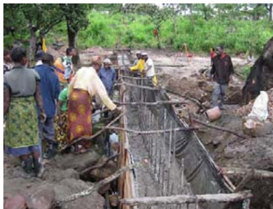
Chinenke irrigation scheme under rehabilitation of the diversion weir. The weir was re-constructed with concrete wall in 2009.
