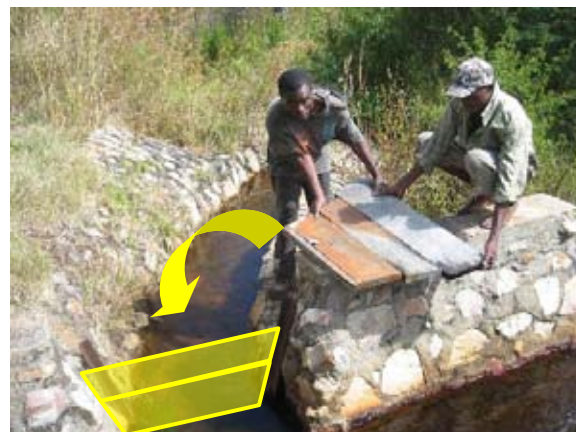
A permanent weir equipped with stop-log gate made of timber board. The farmers operate the gate to adjust water volume for meeting water requirement (June 2009, Chinsali District)
