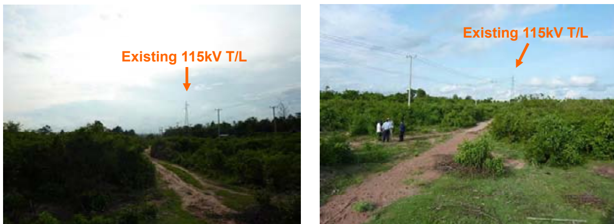
Figure 11-3 Existing 115kV Present Situation around Planned Nongdeun Substation Site (left: Pakbo side, right: Kengkok side)
