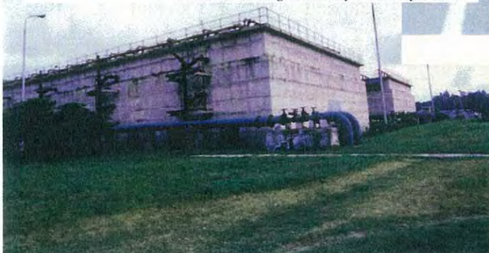
36 MLD UASB Reactor at Kanpur
