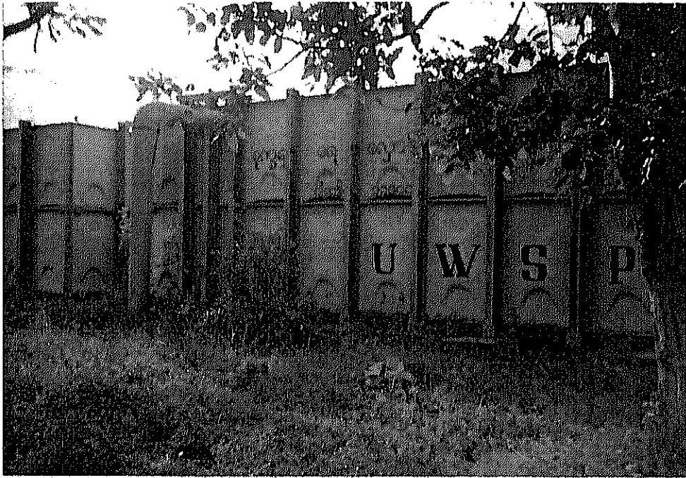
TWO GROUND F.R.P TANKS OF EACH 150 M 3 CAPACITY INSTALLED ON ONE OF THE HIGH LAND PART OF PYAY
