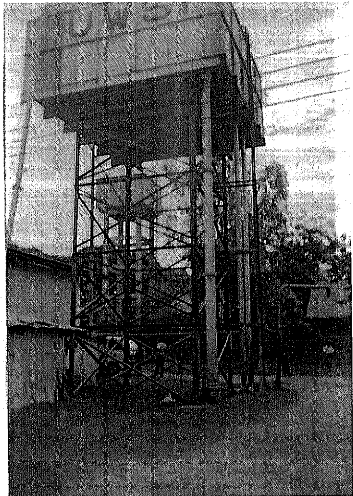
ELEVATED F.R.P TANK OF 20000. GALLONS CAPACITY MAINTAINED BY THE G.A.D.
