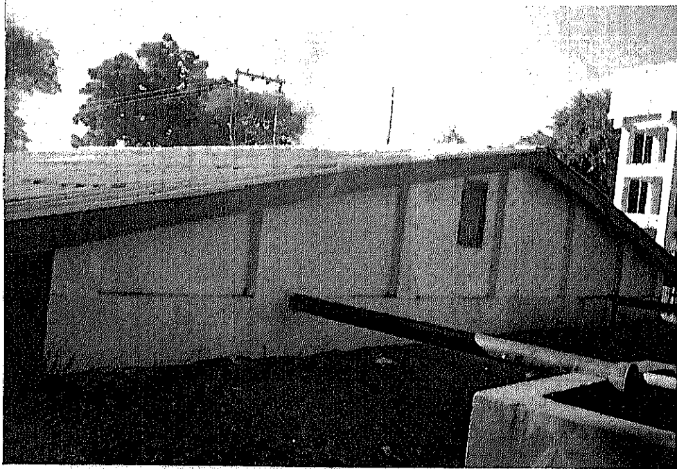
GROUND RESERVOIR OF 315 M 3 CAPACITY
