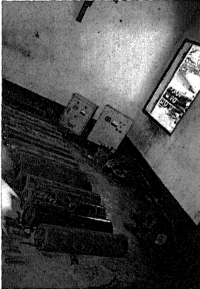
UNSERVICEABLE SUBMERSIBLE PUMPS AND CONTROL PANELS.
