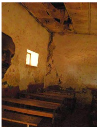
A dilapidated classroom
