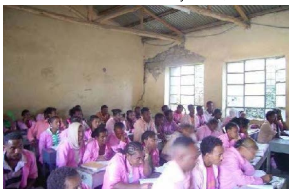
A classroom is dilapidated and in dangerous condition.
