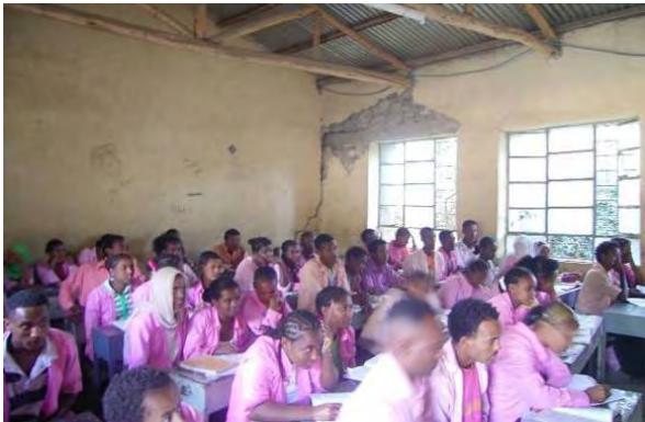
A classroom is dilapidated and in dangerous condition.
