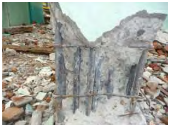
Fig-89: Lap at bottom of column
