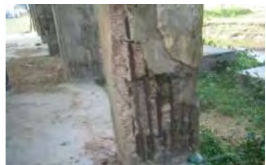
Fig-3 Damaged column by salty
