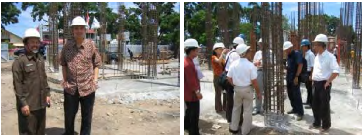
Photo 1. Field trip at school construction site. (left: The president of the department of education in West Sumatra Province and the vice president of the Ministry of Education, and right: the vice mayor of Padang City, specialists, and others)
