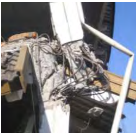
Fig-88: Destruction column and Beam
