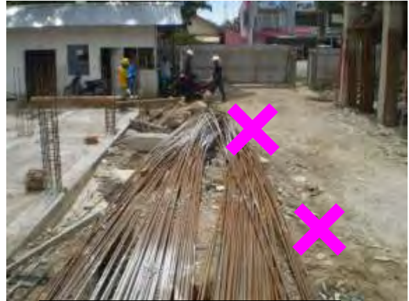
Fig-125 Incorrect stock
