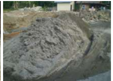
Aggregate left on the ground
