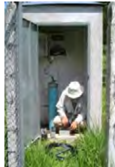
Photo 12 : Monitoring Equipment & Well (WT-4)
