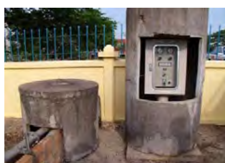
Photo 8 : SRWSA Production Well (PW-4) & Control Box
