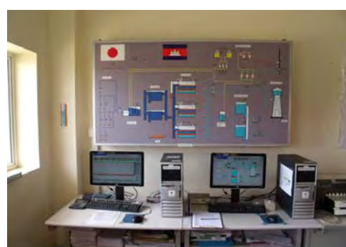
Photo 6: Control Room (Check of Operating Condition of SRWSA Production Wells)
