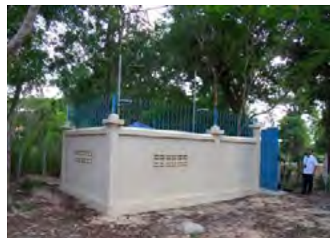
Photo 14: Kravan Monitoring Well (Completion Date: October 2009)
