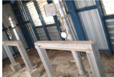
Photo 10: Monitoring Facility of Land subsidence and Groundwater Level
