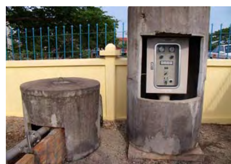
Photo 8 : SRWSA Production Well (PW-4) & Control Box
