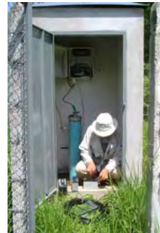
Photo 12 : Monitoring Equipment & Well (WT-4)
