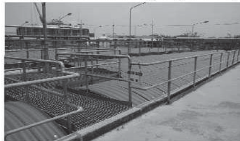
Nong Khaem WWTP (in operation) 1
