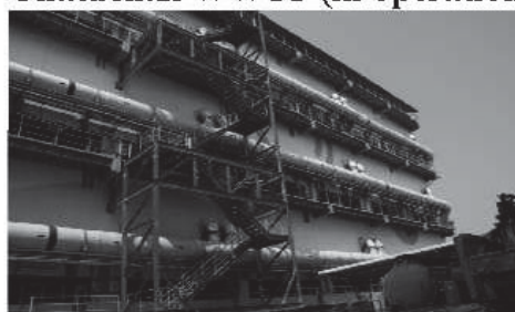
Chatuchak WWTP (in operation)
