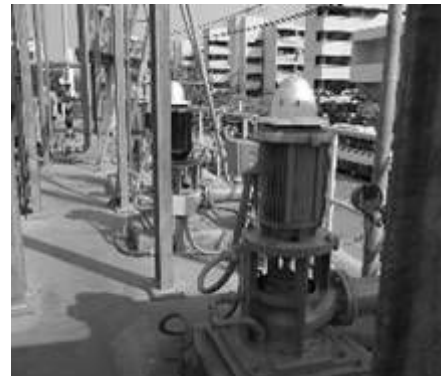
Pump for reuse of treated effluent
