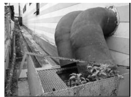
Outlet pipes (bypass discharge)
