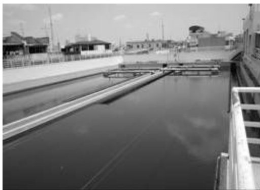
Final sedimentation tank
