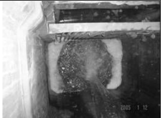
Inside of interceptor chamber
