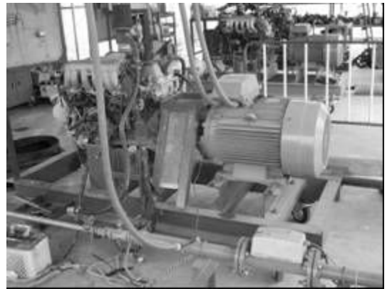
Gas electric generator (truck engine)
