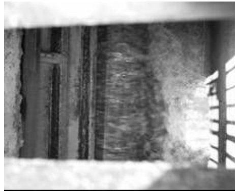
Overflow from interceptor chamber
