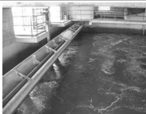
Reactor (supernatant collecting device)
