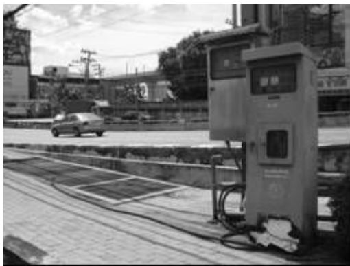
Photo 4.2.7 Existing Manhole Pump (Phetchaburi Street)
