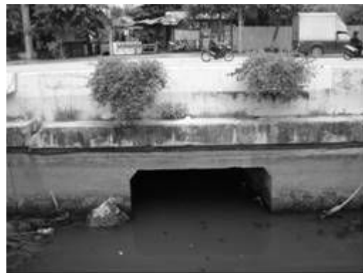
Photo 4.2.6 Outlet Pipe in Dry Weather 4 (June 29 2010, Chong Nonsi Area)
