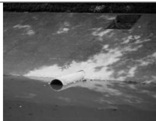
Photo 3.6.4 Drain Pipe under Water
