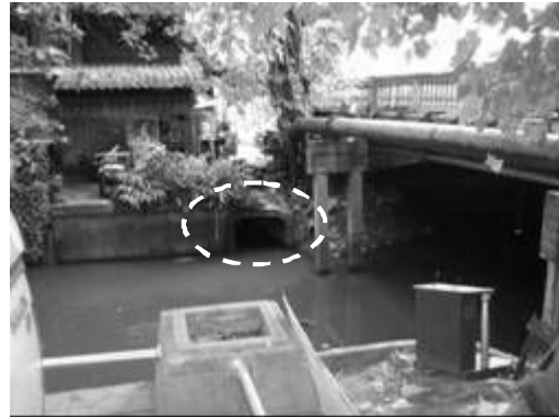
Photo 4.2.4 Outlet Pipe in Dry Weather 2 (June 29 2010, Rattanakosin Treatment Area)
