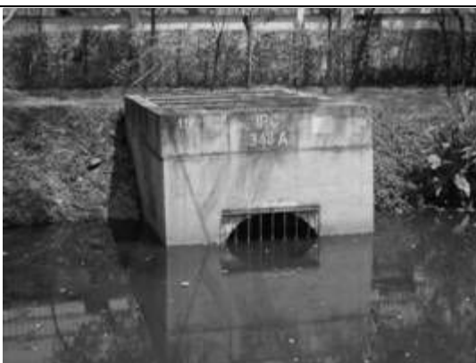
Photo 3.6.3 Interceptor under Water
