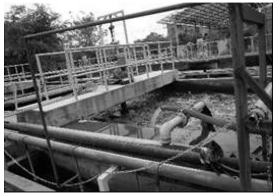
Photo 3.4.12 Reactor (Quicklime Addition)
