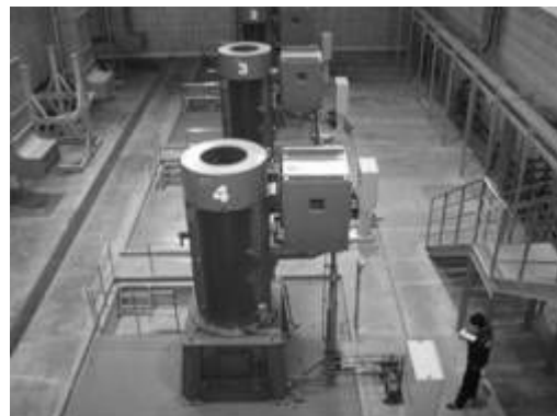
Photo 3.4.8 Pump Pit of No.7 Makkasan Tunnel Pumping Station
