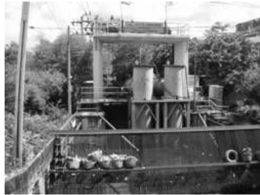
Photo 3.4.4 Existing Storm Water Pumping Station ( along Phetchaburi Street )
