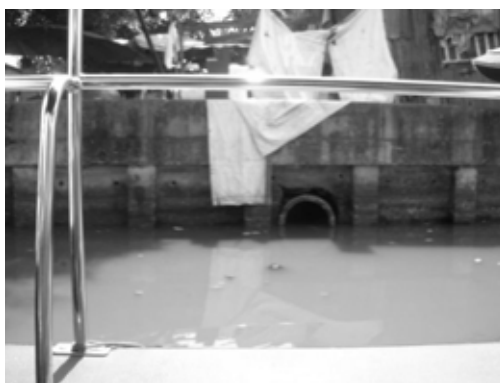
Photo A.3.6 Drainage Pipe
