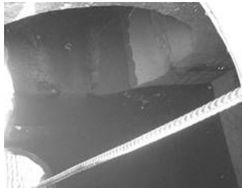
Manhole ( infiltration of klong water )
