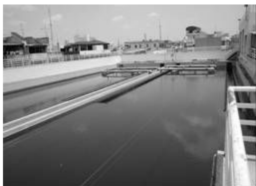
Final sedimentation tank
