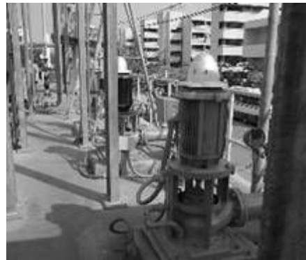
Pump for reuse of treated effluent
