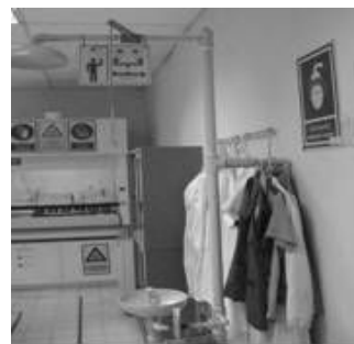
Washing equipment for chemical exposure
