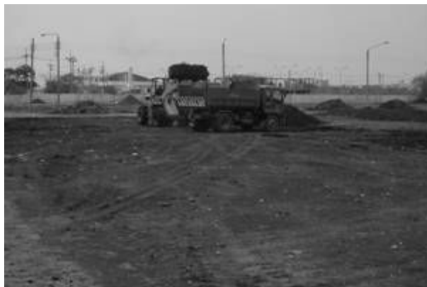
Carrying out of sludge compost
