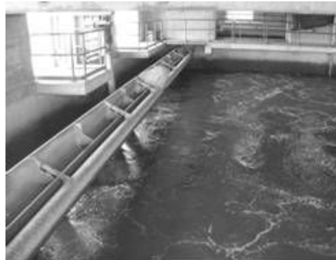
Reactor (supernatant collecting device)
