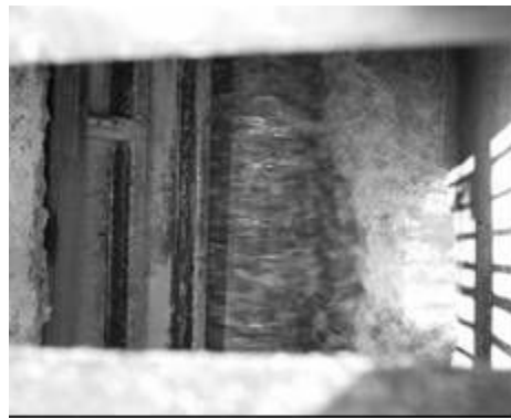
Overflow from interceptor chamber
