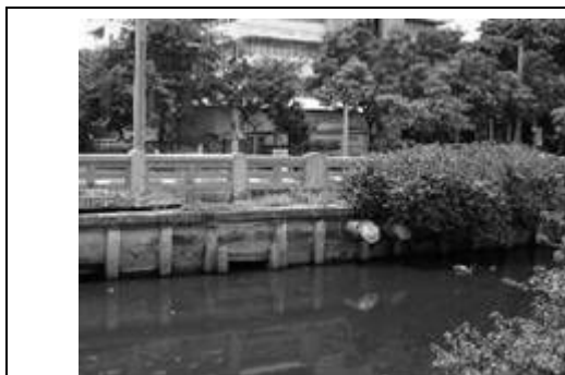
Submerged outlet pipe, pumping station
