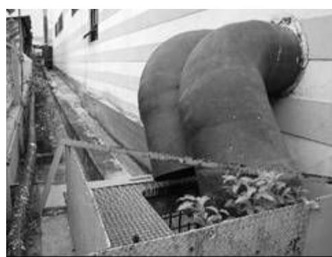
Outlet pipes (bypass discharge)
