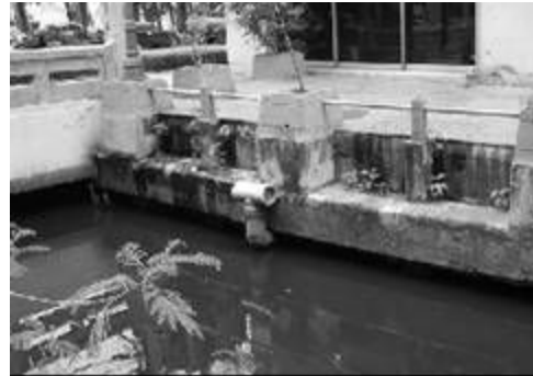
Ventilation for drainage pipe
