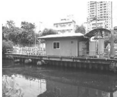
Storm water pumping station
