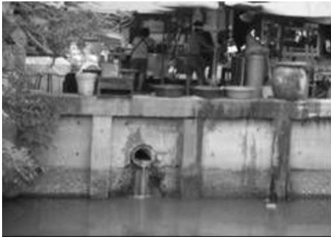
Nontreated wastewater discharge from neighboring treatment area
