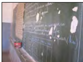
Photo 8 Blackboard with Damage Surface
