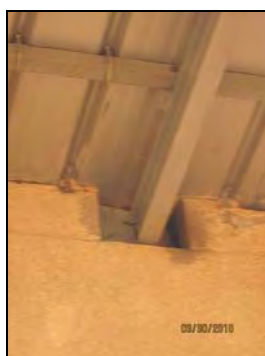
Photo 3 Narrow gap observed between the joist and the wall (Konni Department, Tahoua Region)
