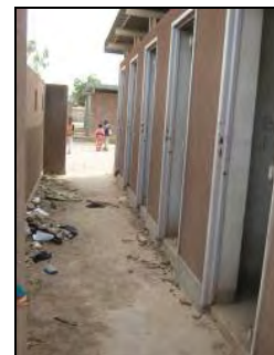
Photo 9 Filthy Latrine Building
