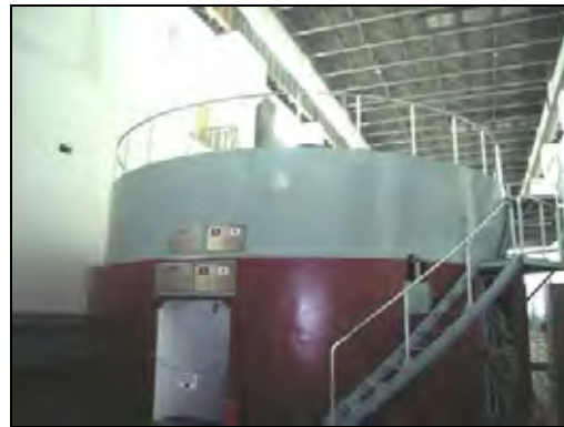
Water Turbine Generator (Unit No. 1)
