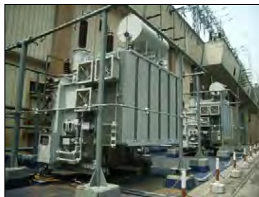
Photo 2: Main Transformers (the Unit No. 1)
