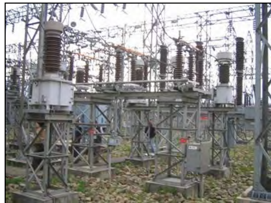
Photo 1: Overview of Equipment in Siuchatar Substation
