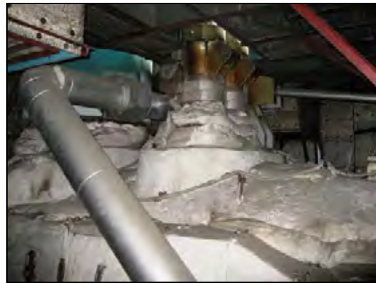
Photo 2: Inside of Steam Turbine of Unit 3 (Steam Valve)
