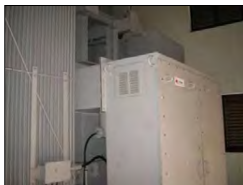
Photo 2: Transformer in K3 Substation
