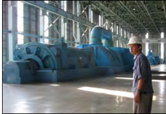
Steam Turbine of Units 3 & 4
