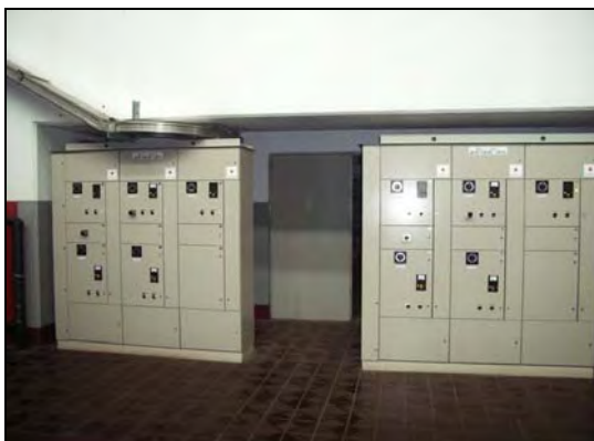
Photo 1: Motor Control Center
