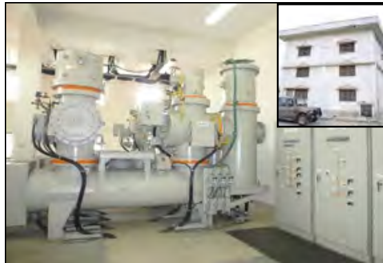
Gas Insulation Switch (GIS) and K3 Substation building
