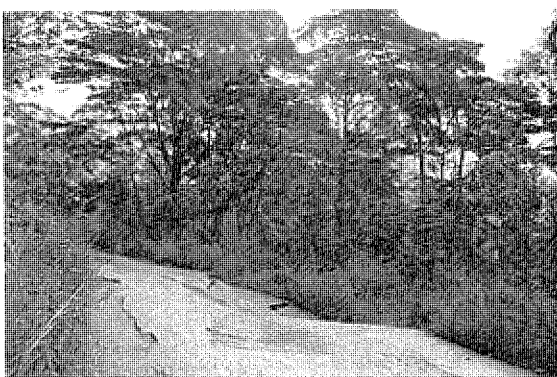
A road with surface damage
