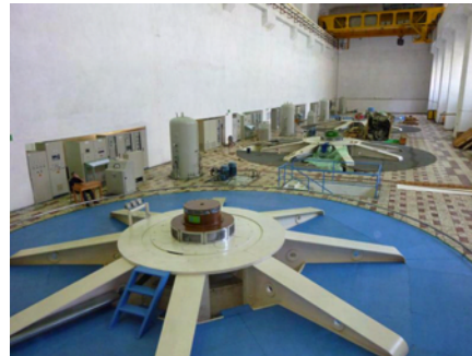
Figure 3: Generator Units (Fierza Hydropower Station)
