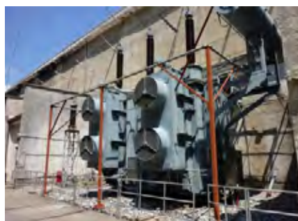
Figure 9: Generator Step-up Transformer 23 (Adjacent to Power Generation Building at Fierza Hydropower Station)
