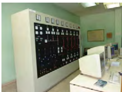
Figure 8: Control Room (Fierza Hydropower Station)
