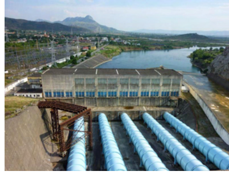
Figure 5: Pipelines (bottom), Power Generation Building (center), and Substation Facilities (upper left) (Vau i Dejes Hydropower Station)
