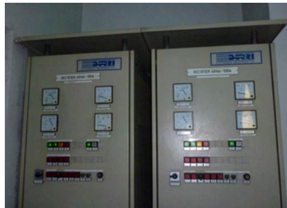
Figure 7: Electrical Equipment Rehabilitated by JICA Loan (Vau i Dejes Hydropower Station)
