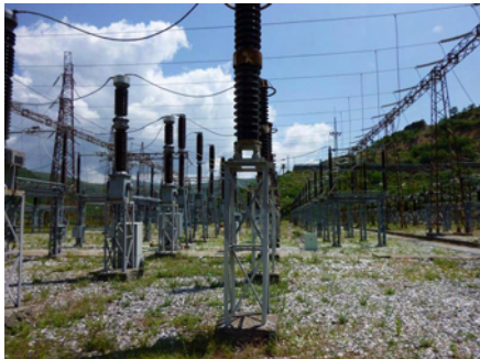
Figure 2: 220KV Isolator Switches (Fierza Hydropower Station)
