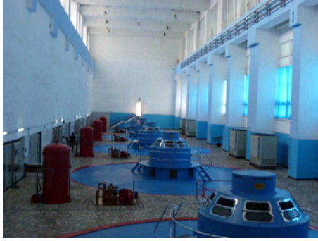
Figure 4: Generator Units (Vau i Dejes Hydropower Station)
