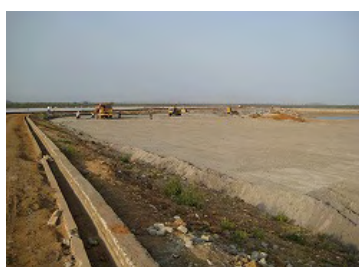
Ash Handling Plant (Ash Dyke)
