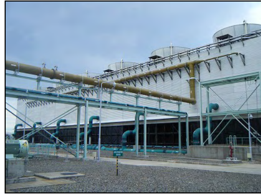
Northern Negros Geothermal Power Plant
