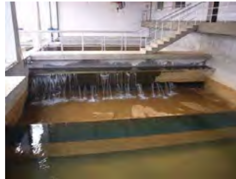
Jian (Wuyueguan Water Plant) Filter Basin
