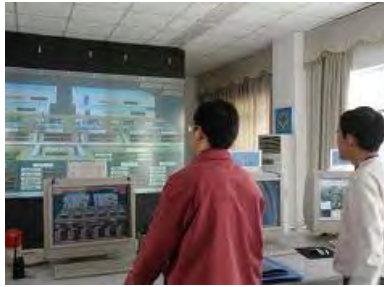
Monitoring room at Sanjin Water Plant in Nanning City
