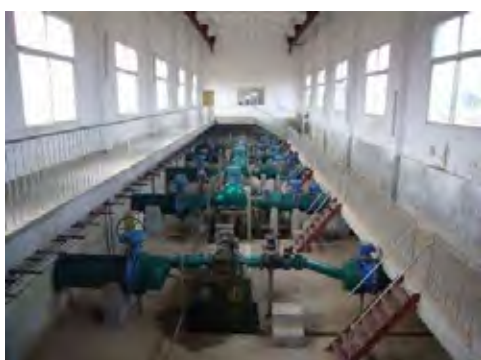
Distribution Pumps in No. 3 Water Plant in Ganzhou
