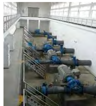
Guilin Chengbei Water Plant Pumps for transmission
