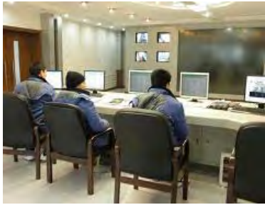
Monitoring room at Chengbei Water Plant in Guilin City
