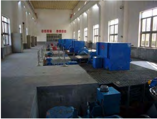
No.8 Water Plant Distribution Facility
