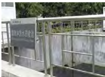
Water recycling pond at Sanjin Water Plant in Nanning
