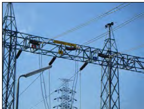
115kV transmission line constructed by the project
