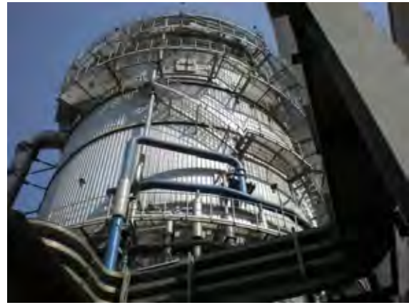
Fig. 12: Smoke elimination/desulphurization equipment
