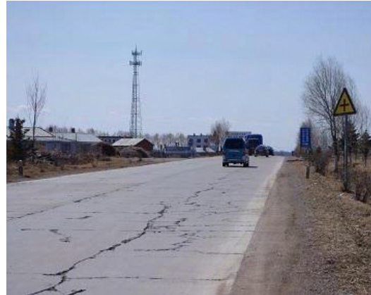
Fig. 14 Cracks on Road Surface
