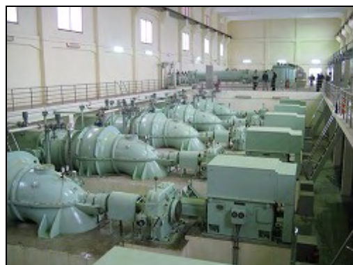
Yen So Pumping Station
