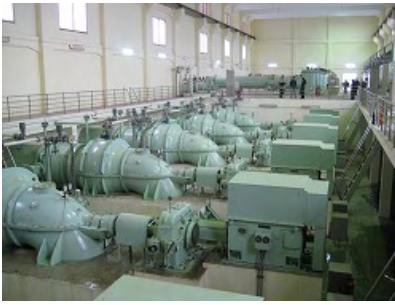
Yen So Pumping Station
