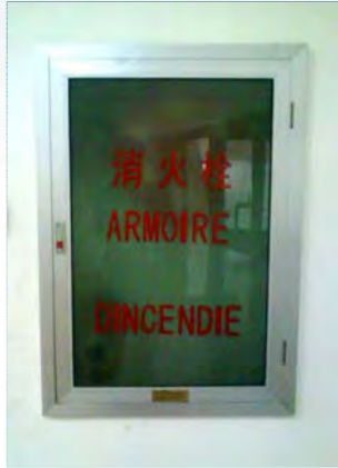
Cotonou (Benin) International Congress Center Fire safety device
