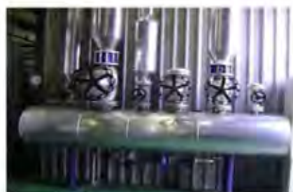
Fig.-6-2 : 8 t/h boiler steam header
