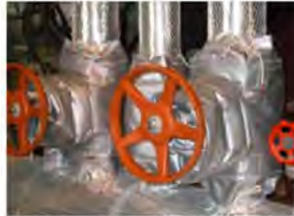
FIG.-6-3 : An Example of Insulation Jacket on Valves
