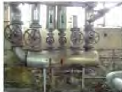
Fig.-6-1 : Steam header
