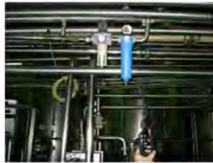
Fig.-5-3 : An Example of Leaking Part
